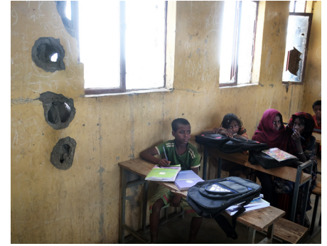
Shrapnel in the classroom.
